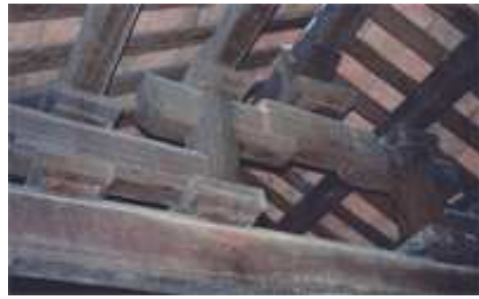
Close-up photo of the interdependent RAFTER and PURLIN set in creating the roof's framework
